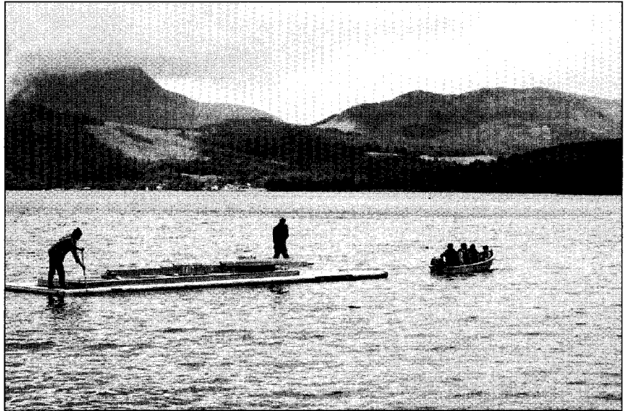
Building a new club - the new rowing pontoon is delivered! Photo courtesy of James Cowderoy
